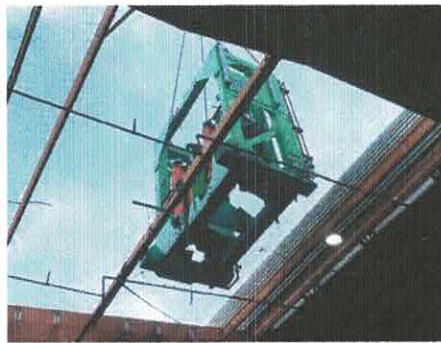
Quad roll log turner being craned in through the roof at Hyne's Tumbarumba mill.
