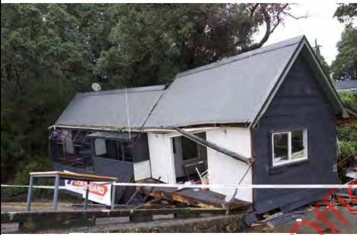
Coastguard Building in French Bay damaged by a slip Source: Stuff.co.nz
