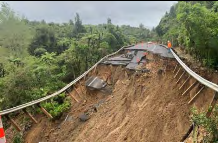
Actively moving slip on SH25A, Coromandel Source: Stuff.co.nz
