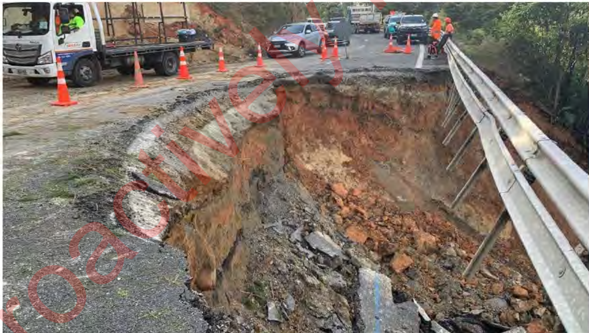
Figure 2: Single lane access on SH25 Waihi to Whangamata (Source: Waka Kotahi 8:17AM 8 March)
