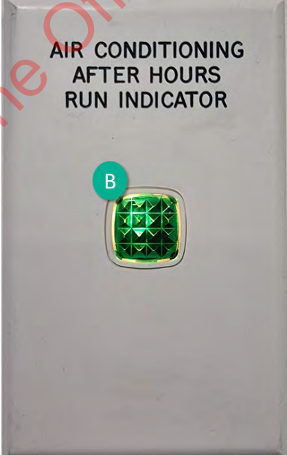
Air conditioning on/off indicator light
