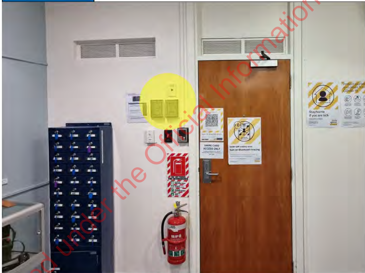
Air conditioning switch location
