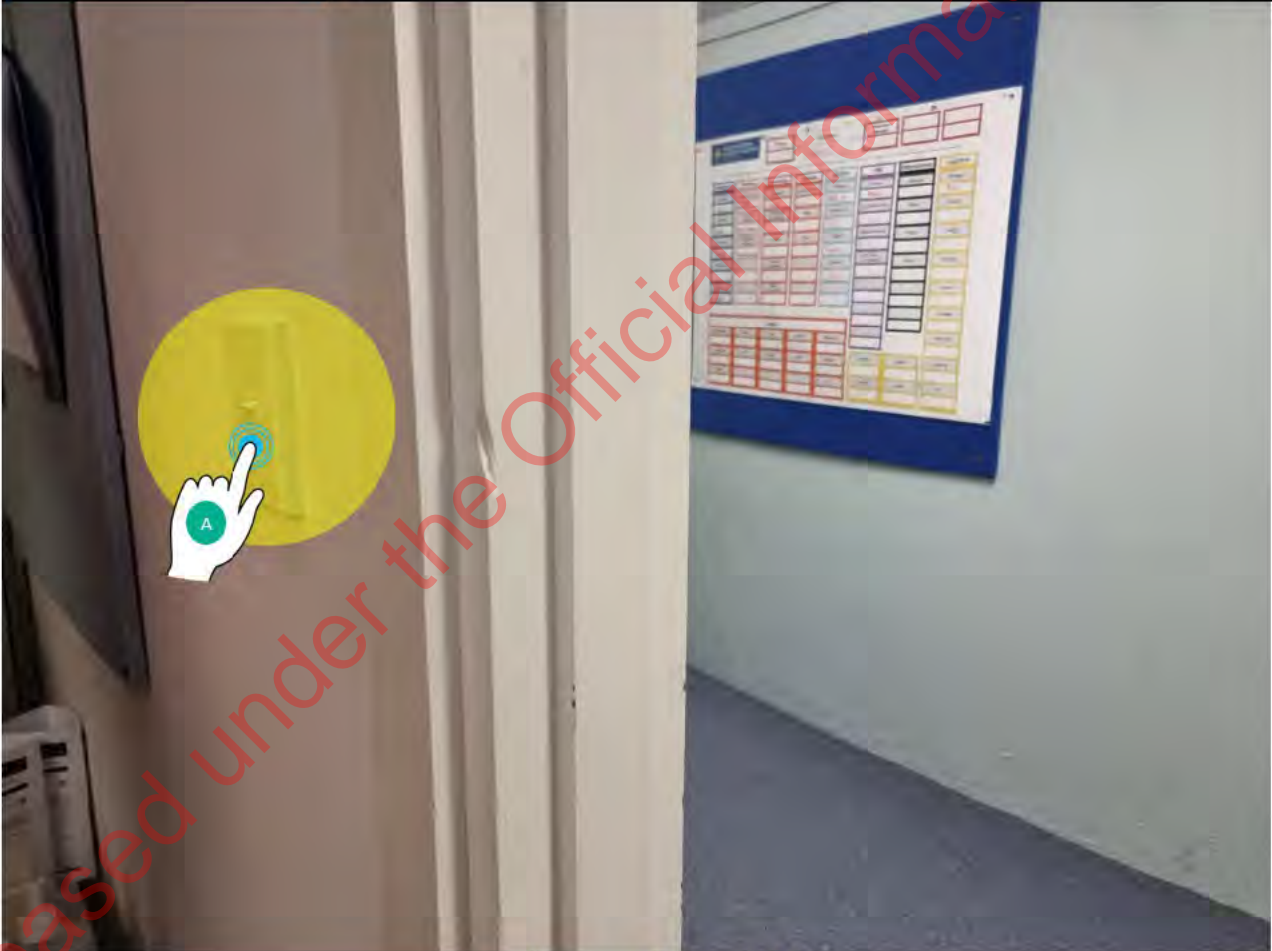
Operations room light switch #1
